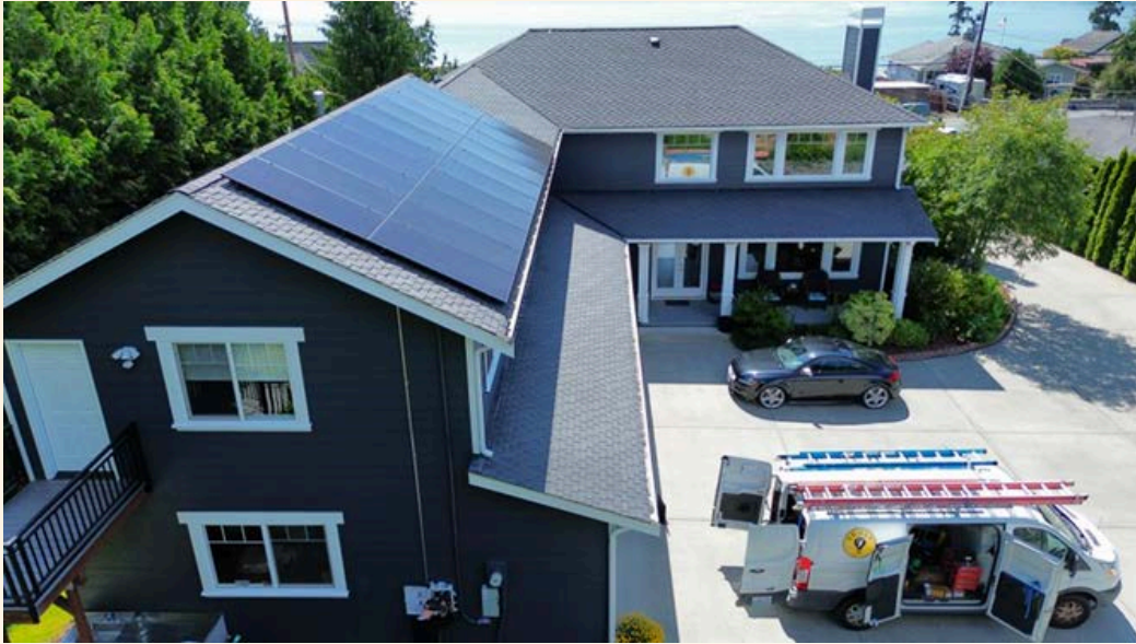
Residential solar installation
