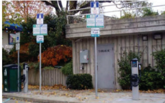
Electric vehicle charging stations at the Marina Parking Lot in downtown Kirkland.
