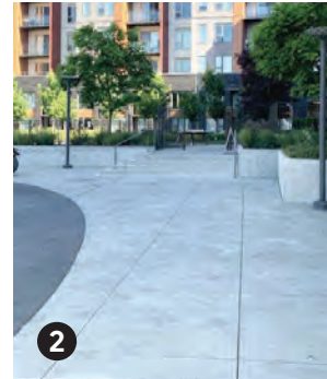
2 Existing PIP concrete
