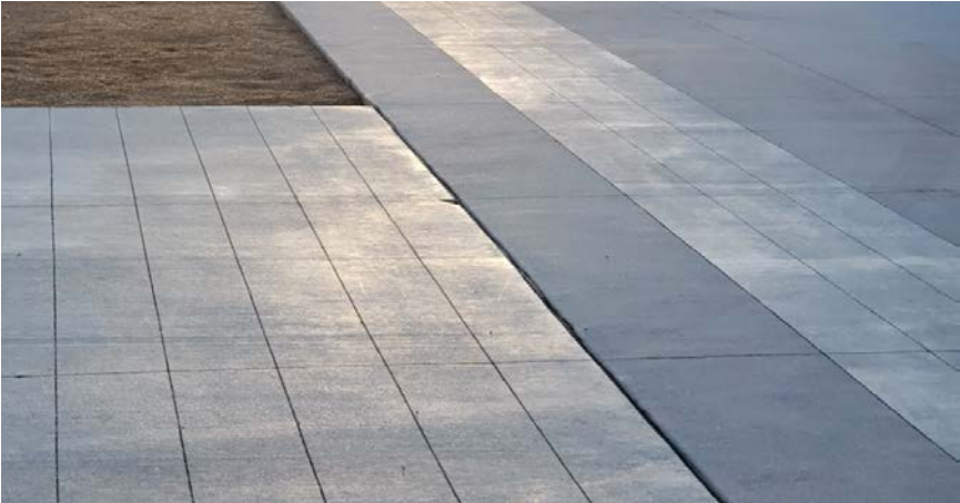
Cast-in-place concrete sidewalks with select areas of special finish such as integral color or unique finish.
