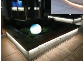
LED Accent Lighting Along Walls and Stairs
