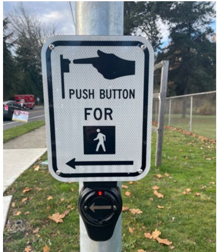
Figure 61. APS Push Button on NE 132nd St
