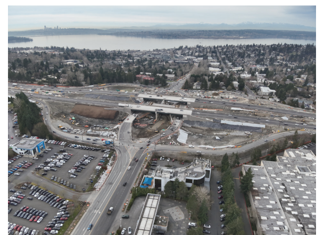
Future site of the Area's bus-rapid transit station at NE 85th Street and I-405.
