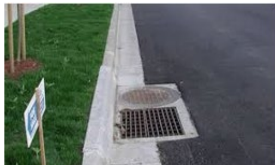
Typical StormFilter in Roadway
