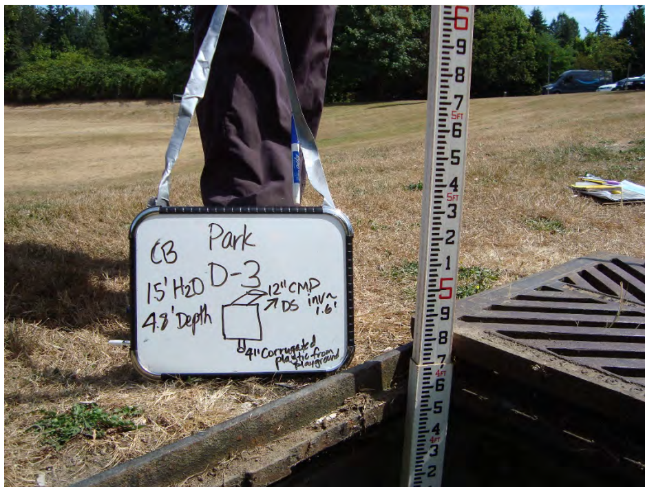
Infrastructure Issue: Curb weep observed flowing into catch basin 10514(SD-3 in photo) from the curb on NE 100 th Street.
