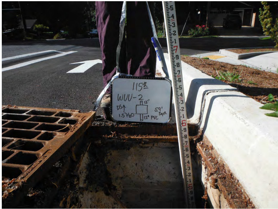
Infrastructure Issue: CB 10170 on the west side of 116 th Ave NE at the intersection with NE 95 th Street is overgrown and inaccessible.
