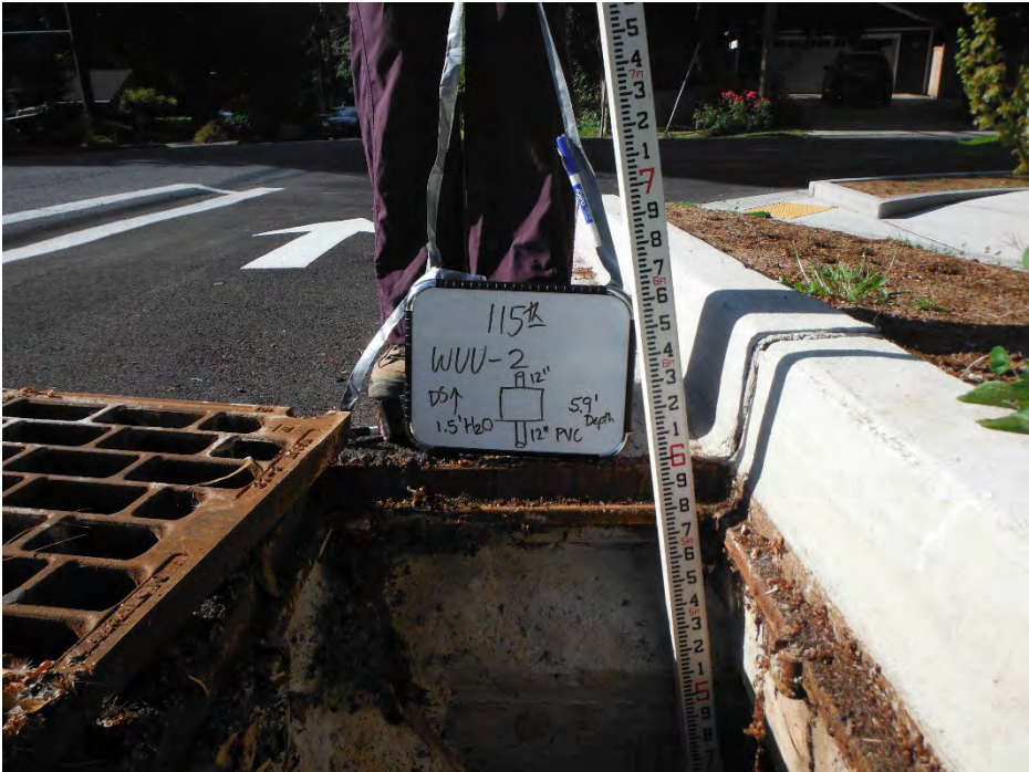
Infrastructure Issue: CB 10170 on the west side of 116 th Ave NE at the intersection with NE 95 th Street is overgrown and inaccessible.
