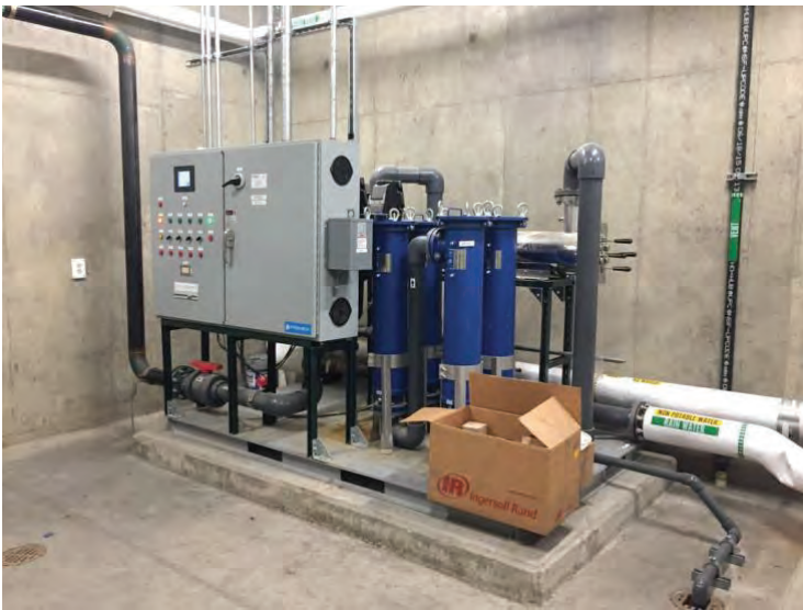
Figure 20 Part of onsite catchment water filtration system.
