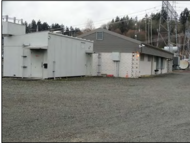
Figure 7-138. The Sammamish Substation in Redmond, view west.
