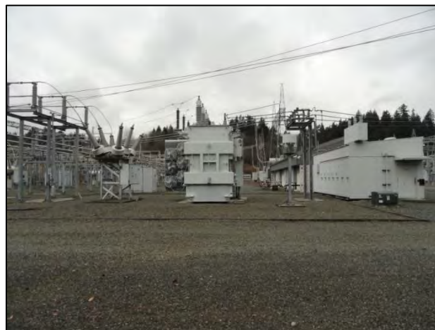
Figure 7-140. Transformer, control house, and bus work at the Sammamish Substation, view west.
