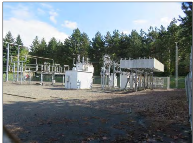
Figure 7-181. PSE substation at 13211 NE 123 rd St., view south.
