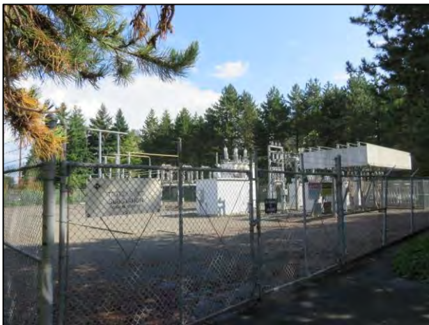
Figure 7-180. PSE substation at 13211 NE 123 rd St., view southeast.
