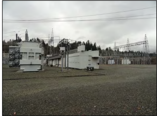
Figure 7-139. Transformer, control house, and bus work at the Sammamish Substation, view northwest
