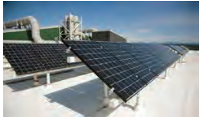
Rooftop solar panels at Bow Lake Recycling and Transfer Station
