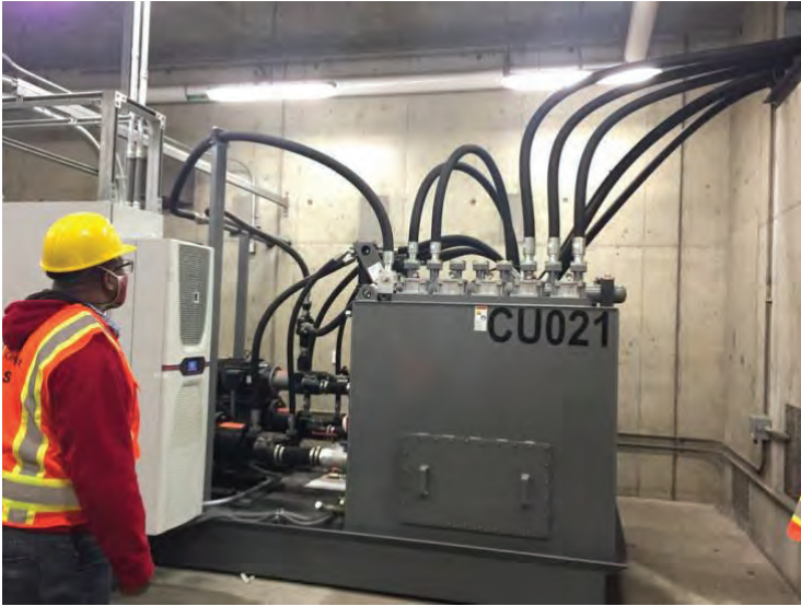
Figure 19 Looking at hydraulics room of the SSI 4500SPH.
