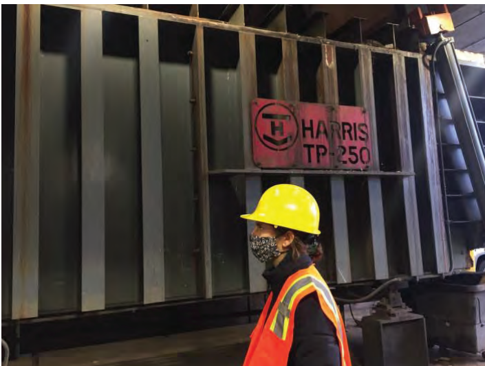
Figure 21 Back-up compactor, the Harris TP-250.
