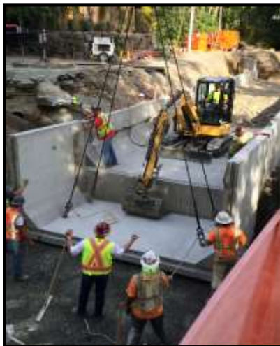
Concrete Culverts with new sediment trap
