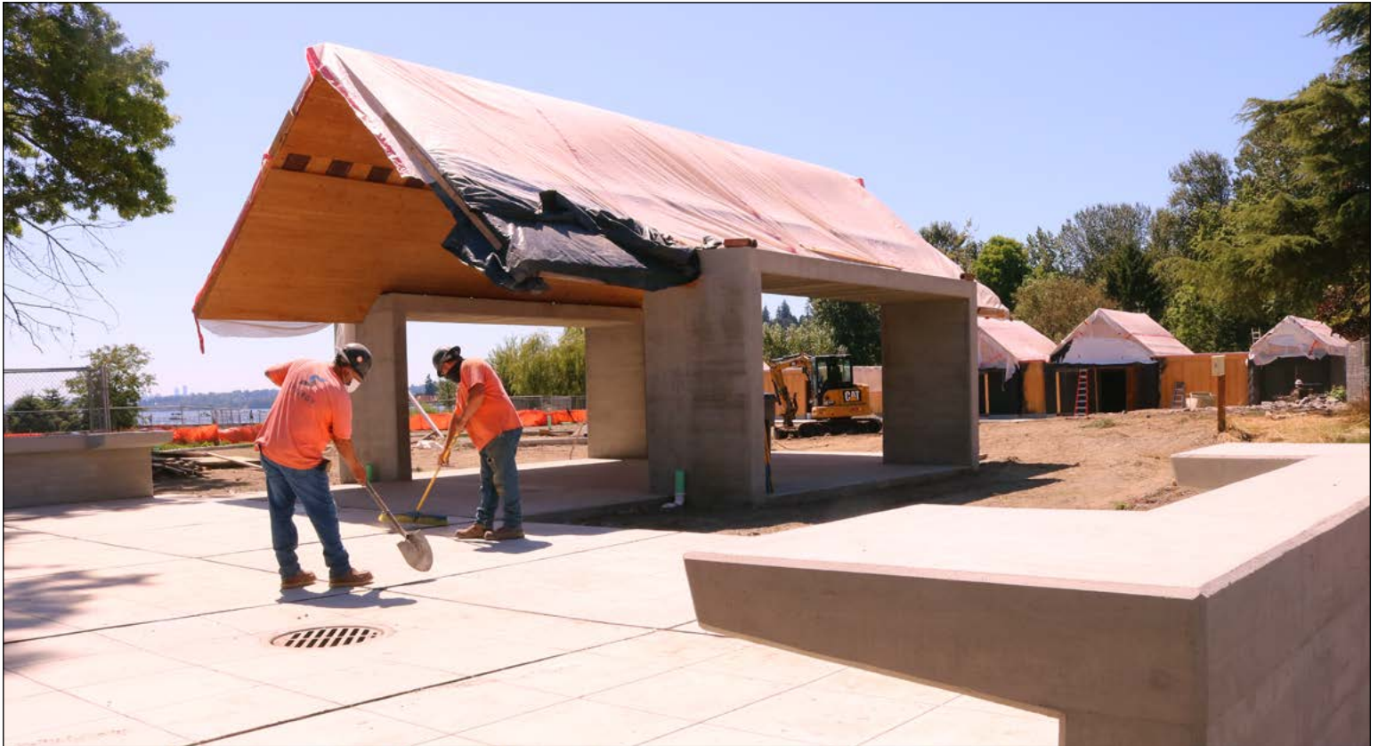
After a day of working in late July’s heat, construction workers from Synergy Construction tidy up the pavilion’s courtyard at Juanita Beach Park. Synergy Construction has been renovating park since mid-January with a pair of picnic pavilions, a bathhouse and a new all-ages-and-all-abilities playground that will feature a new swingset. The contractor expects to complete the renovation by the end of summer.
