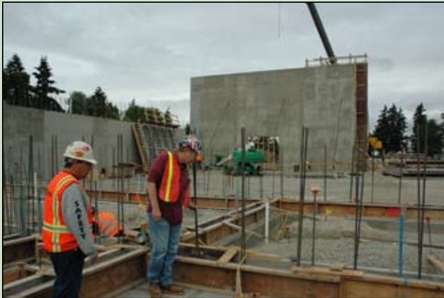
City Building Inspector David Thress (right) inspects the gymnasium stem walls as Assistant Superintendent John Paul (left) looks on.
