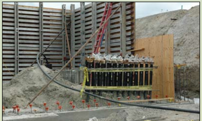
The 30 miles of underground piping for the geothermal systems end into 24 above ground valves.
